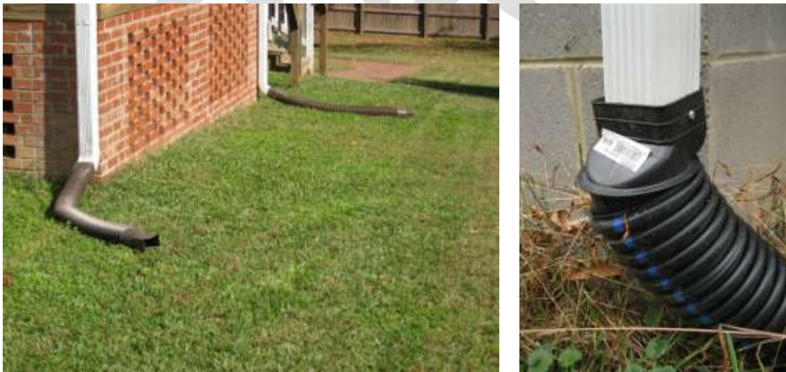
Figure 24-3. Disconnected downspouts on the left and a converter joint on the right (Carmen, NCSU)
