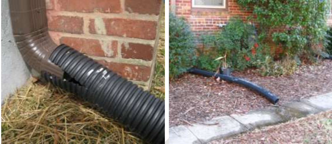
Figure 24-4. Poorly designed and installed downspout disconnections (Carmen, NCSU)
